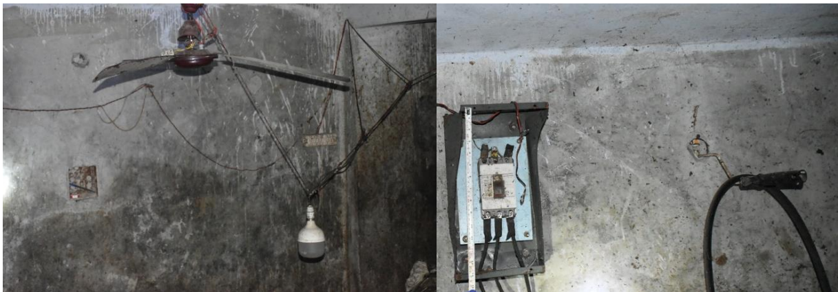
Fig. 3: Photographs showing the cascading burnt impressions on walls in the factory.
